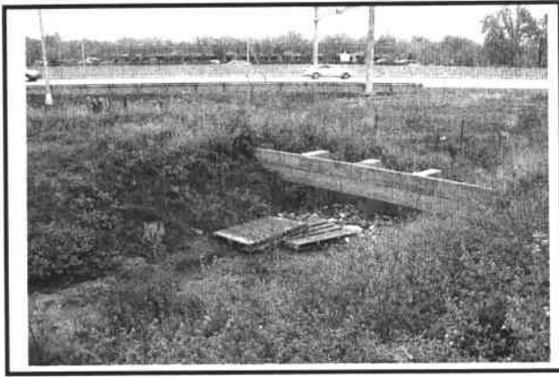
Outlet with debris
