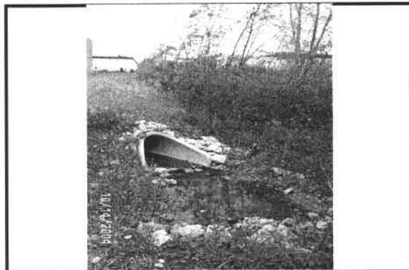
Pond outlet pipe flared end section
