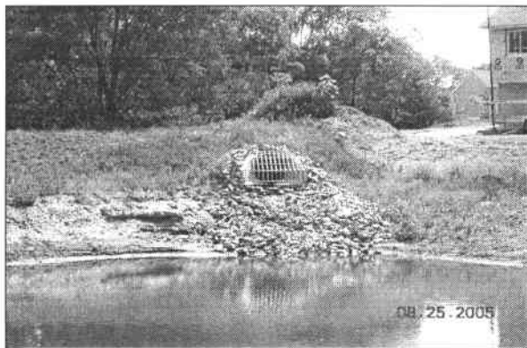
Erosion at southeast inlet
