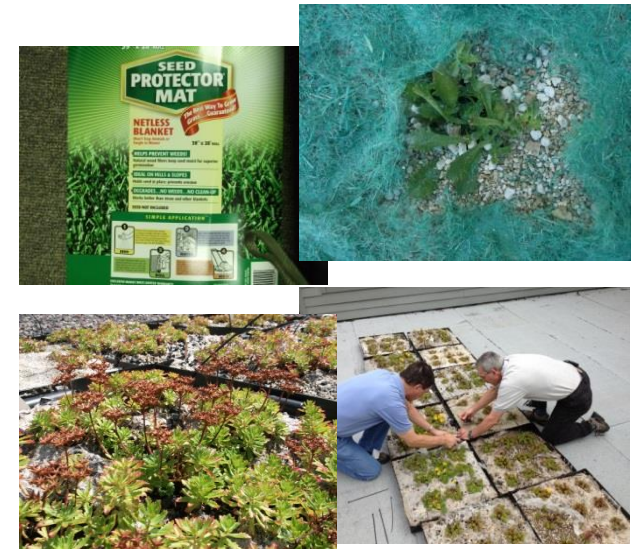
Clockwise from upper left: Protective mat placed on the medium and around a sedum; installation of test modules in 2013; modules in July 2015, two years after installation.
