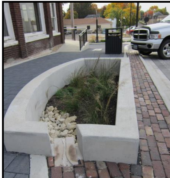
Stormwater Planter in West Union, IA
