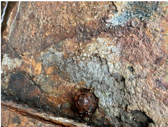
3 – Inner 24-inch panel bolts rust welded.
