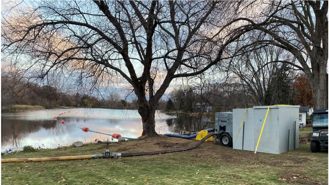
The Meadow Lake pump and enclosure in a resident's backyard at the start, with the intake pipe extending out into the lake.
