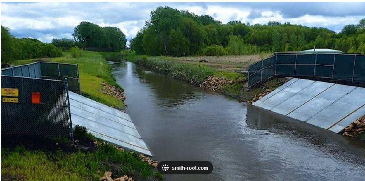
Figure 5. High voltage electric fish barrier (image courtesy of Smith-Root).
