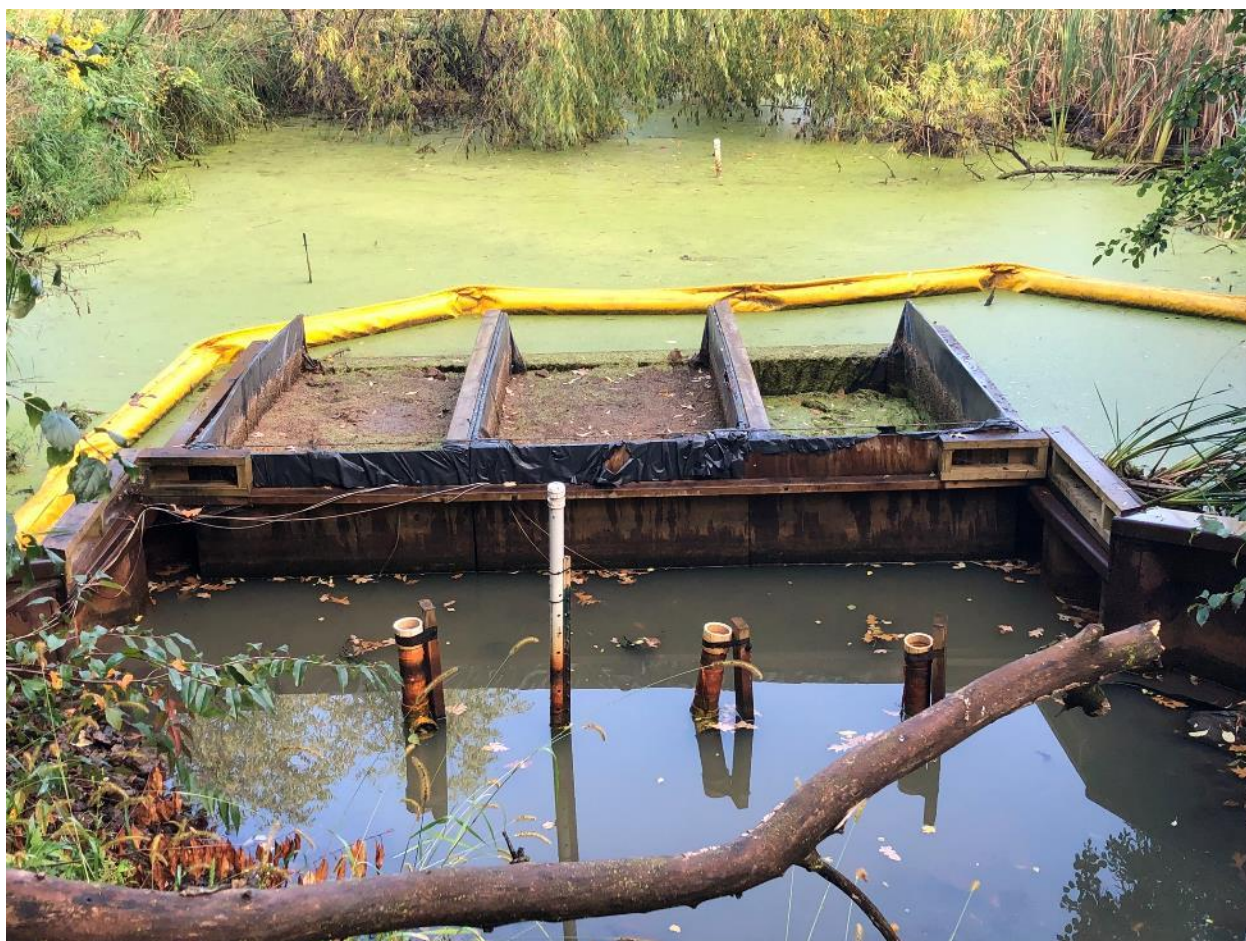
No flow over the weir, the SRP filters are dry.
